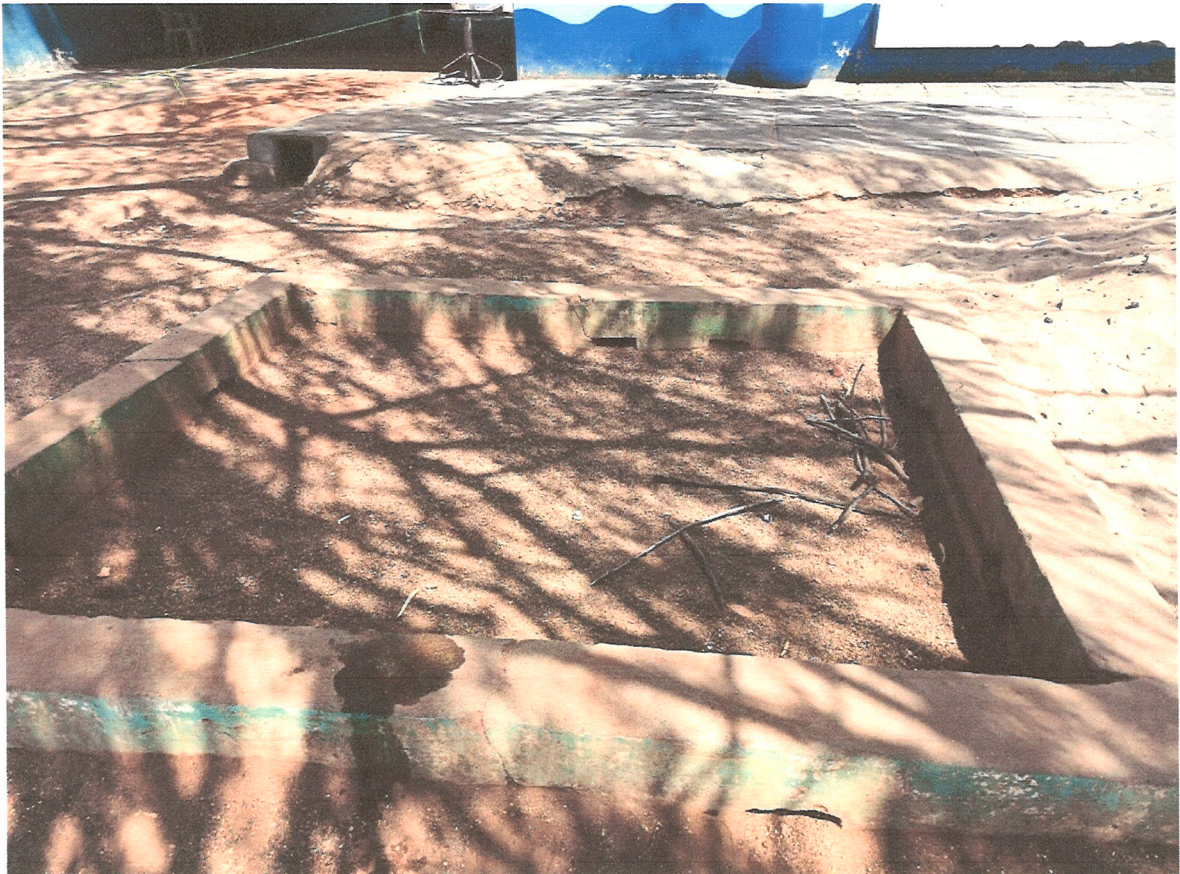
Rain water Harvesting Pit
